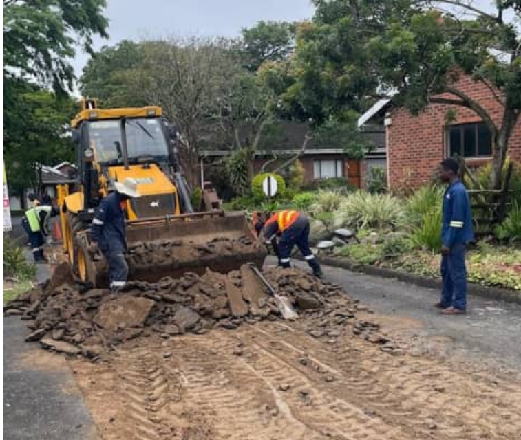
ROADWORKS: The village is full of the hustle and bustle of contractors on site repairing our roads. Estate Manager, Winston vd Schyff said they are expected to be around until mid December. Photo: Don Tandy
